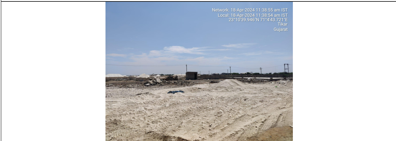
Chem stone Industries - Plant and machinery removed from site. Unit completely dismantled.
