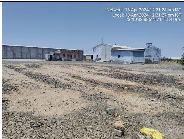
Abd Chemicals - Looking to condition of Plant and machinery, Unit is in non-operation condition since long.
