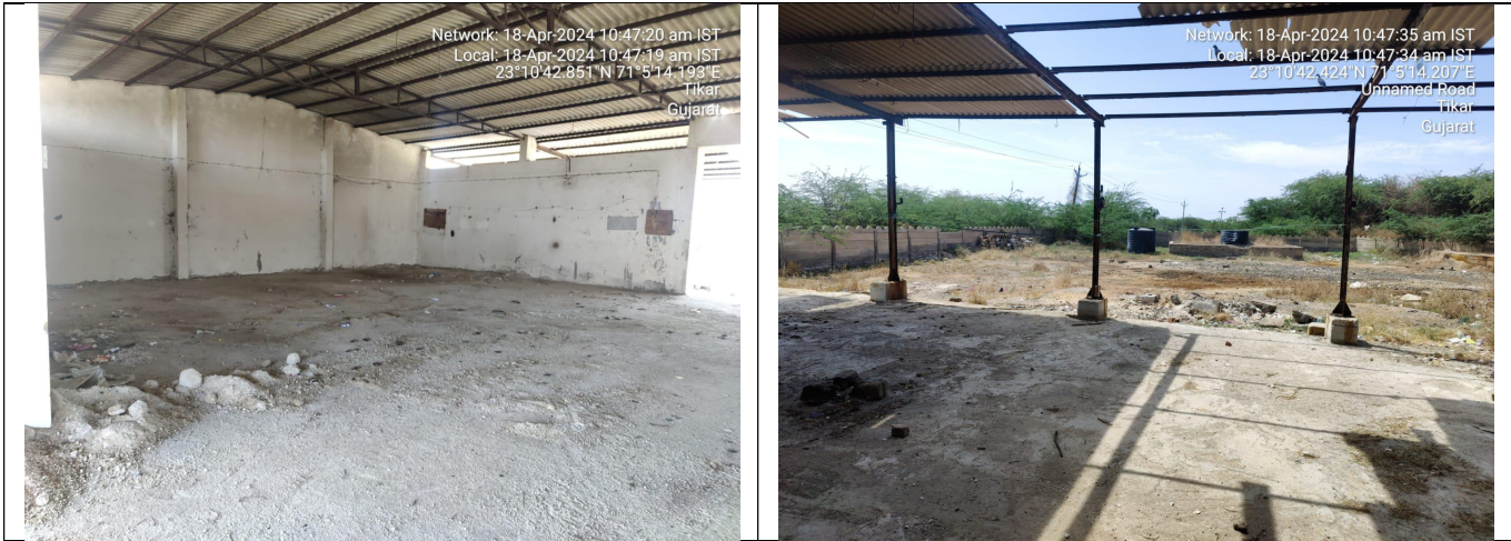
Shiv Krupa Enviro Systems P. L. (Shiv Krupa Chemicals) - Plant and machinery removed from site.
