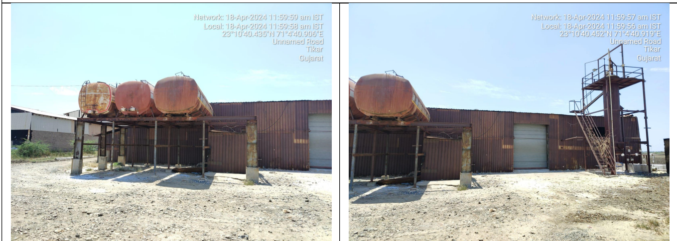
Shiv Industries - Looking to condition of Plant and machinery, Unit is in non-operation condition since long.
